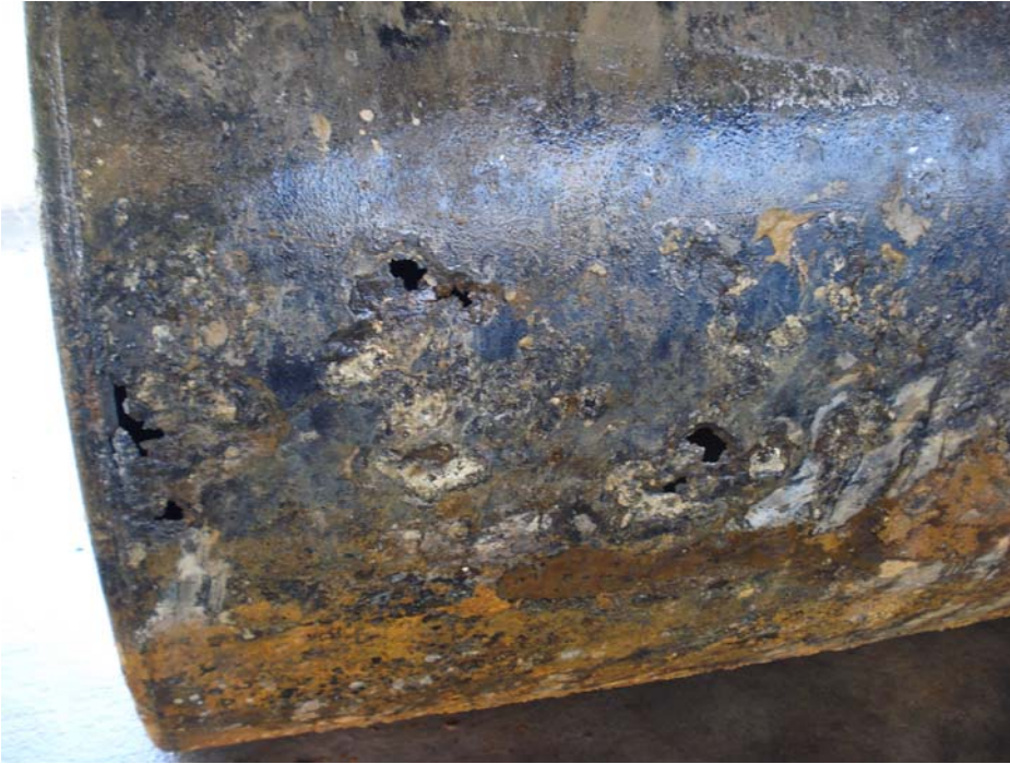
UST TT-2223 Pitting
