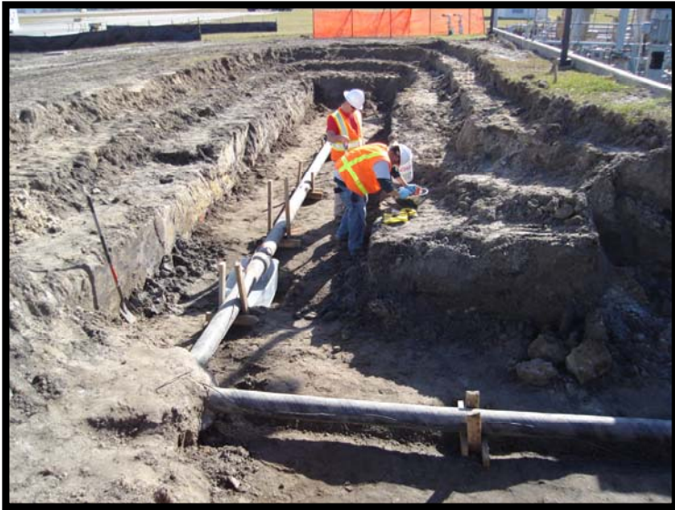
Expose pipe leak location at tracer probes 196, 200, & 201
