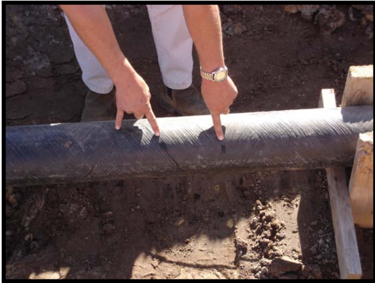
Leaks on pipe at tracer probes 184 & 185
