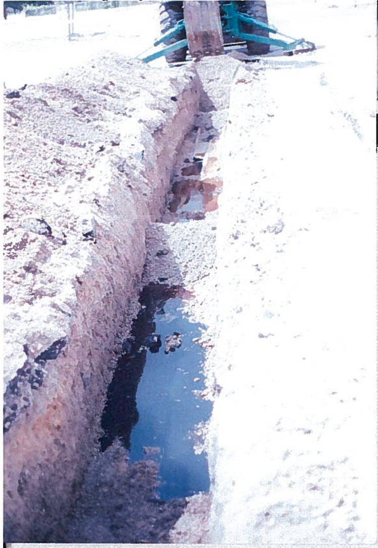
Photo #6 Free product in fuel supply line trench
