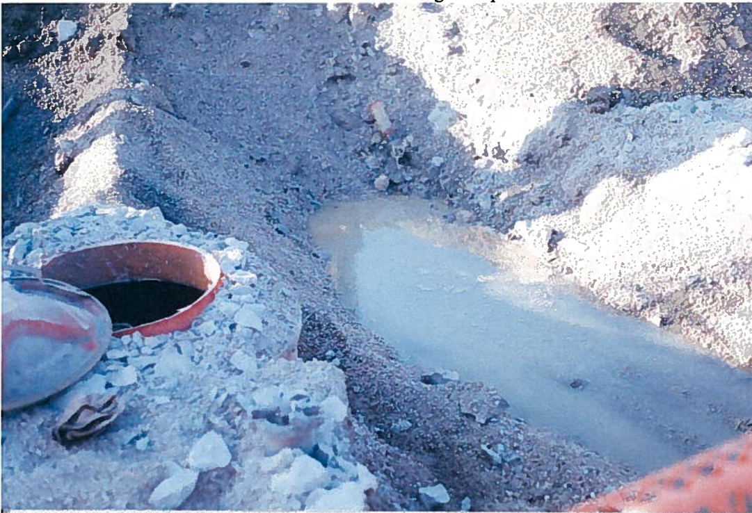
Photo #2 Groundwater in the excavation pit.
