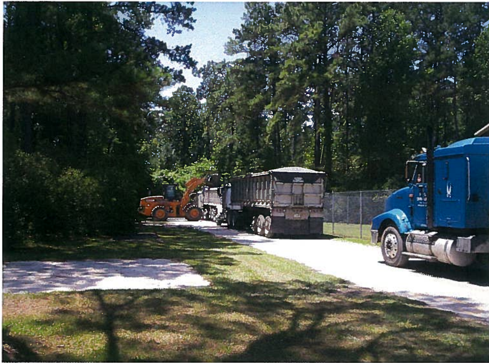
Photo 7; TP-467 Soil stockpile being loaded prior to weighing. A total of 578.78 Tons was transported to the soil disposal facility from this drying pad.
