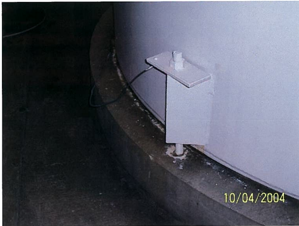
Anchor Bolt and Grounding Cable
