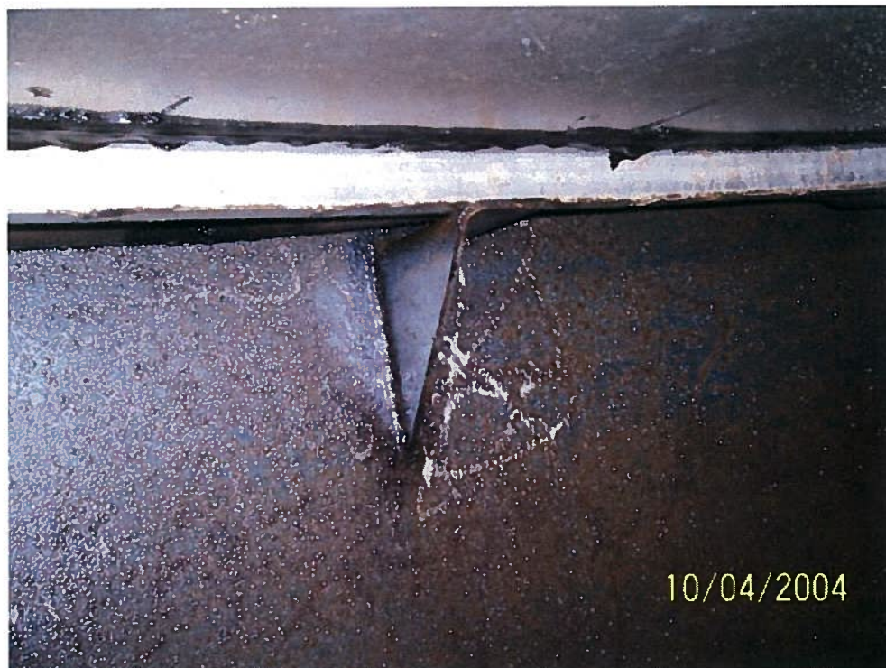
Floating Roof Low Position Support
