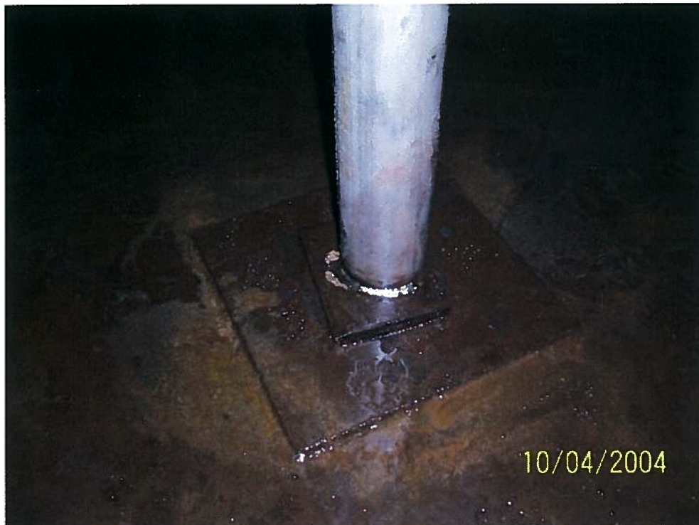
Fixed Roof Support/Gauge Well
