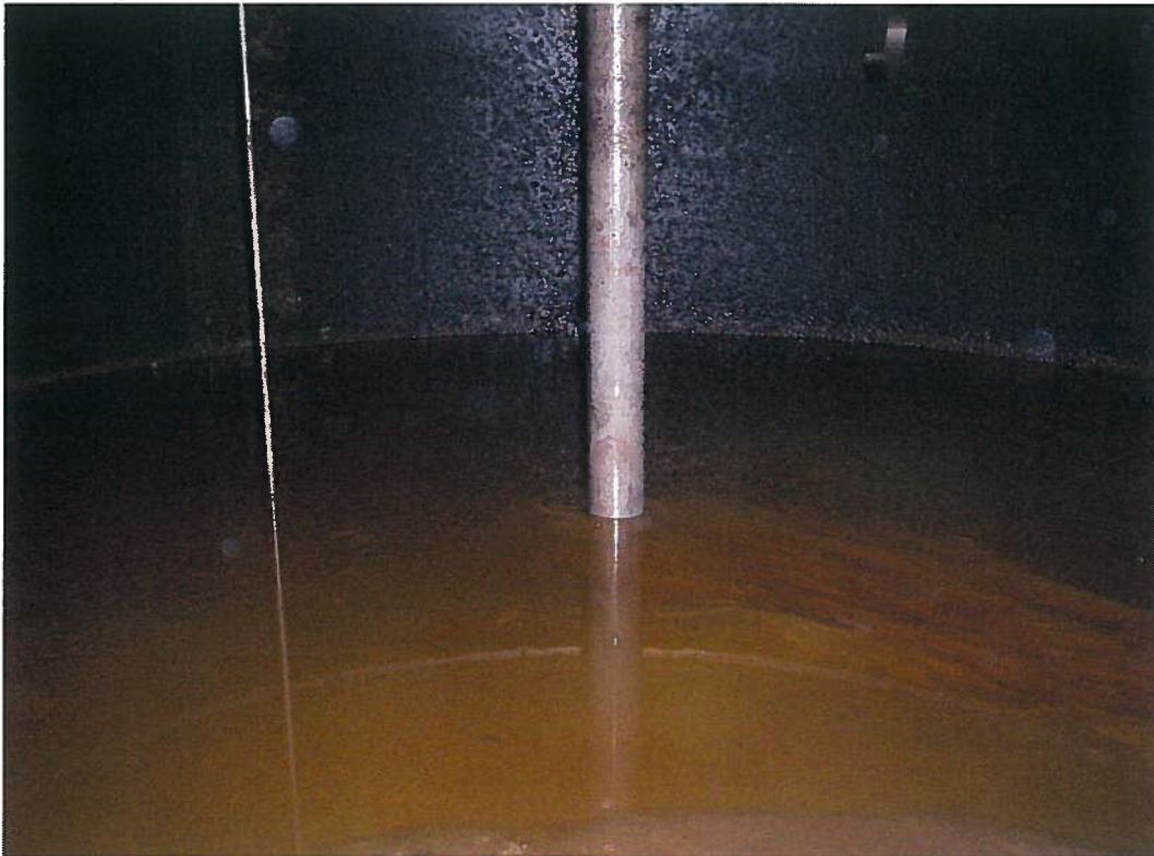
Photo 4; Sludge remaining after fuel removed from the AST.
