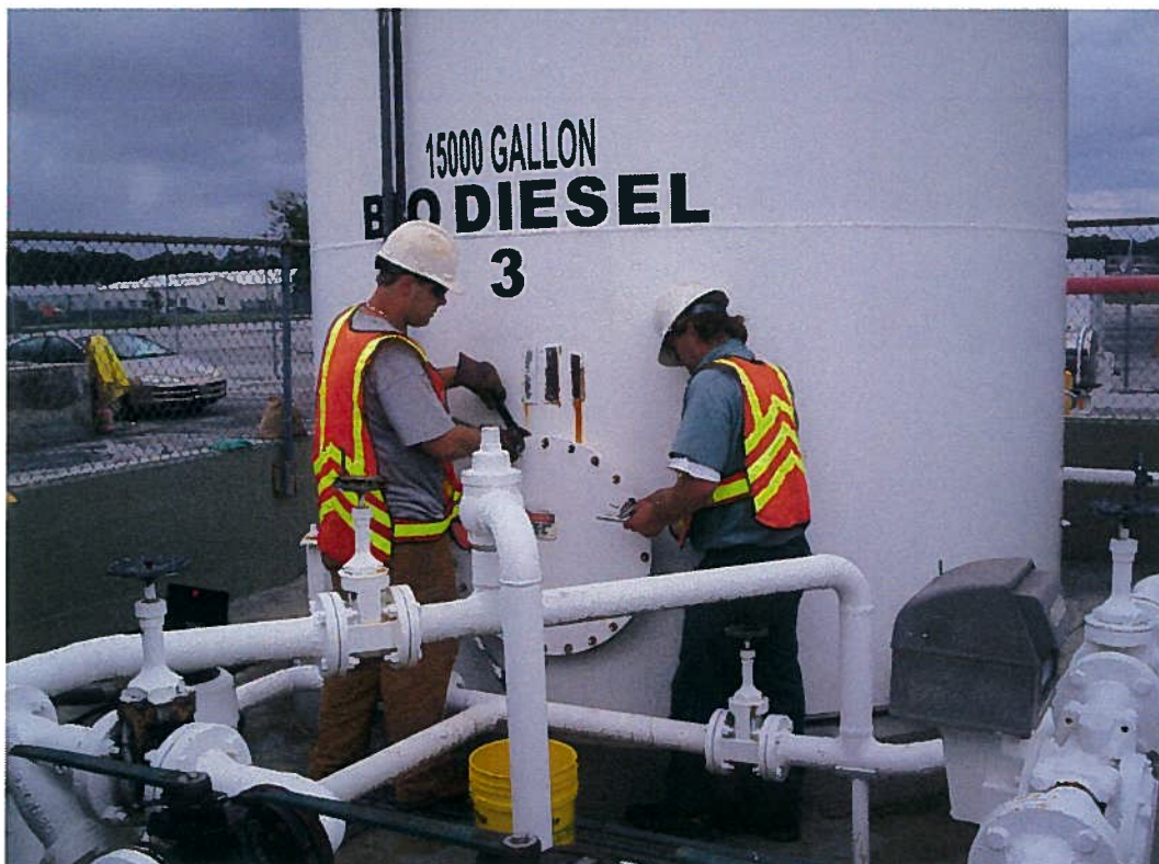
Photo 16; Completion of cleaning with installation of man ways using new gaskets and new nuts and bolts
