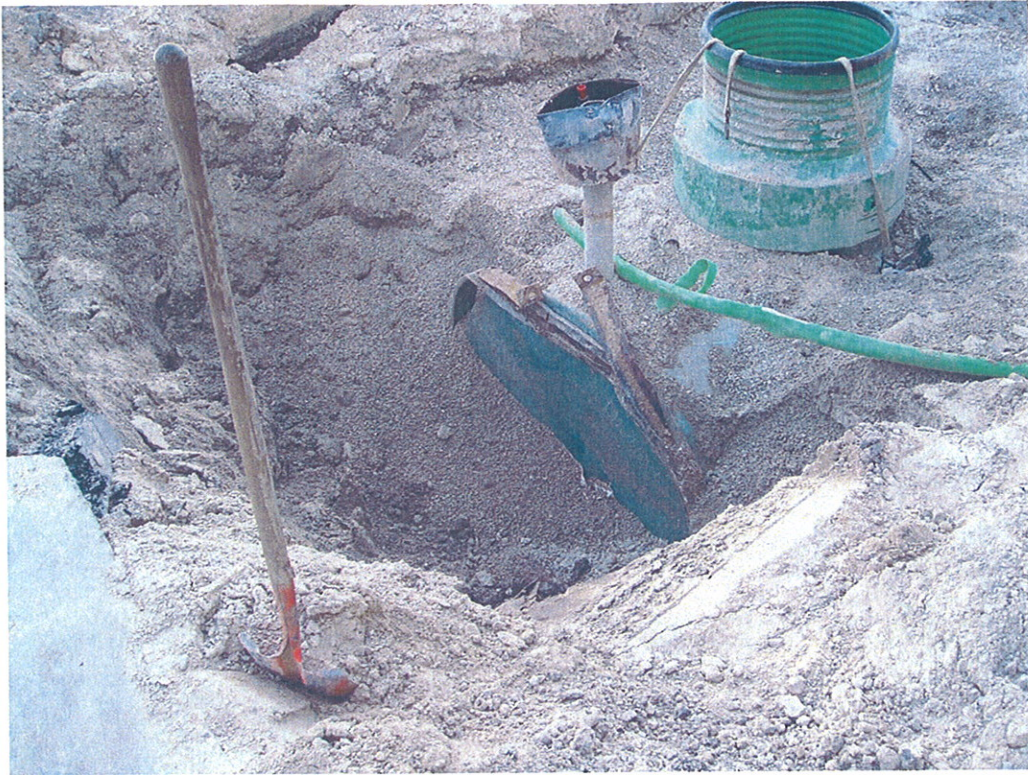
Building AS-4159 UST Exposed
