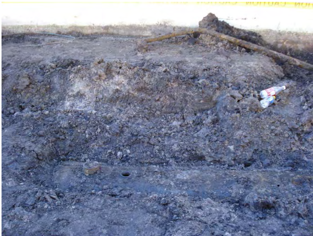
UST TT-3026 – Tarawa Terrace – Tank Exposed Pic #2 24Oct08
