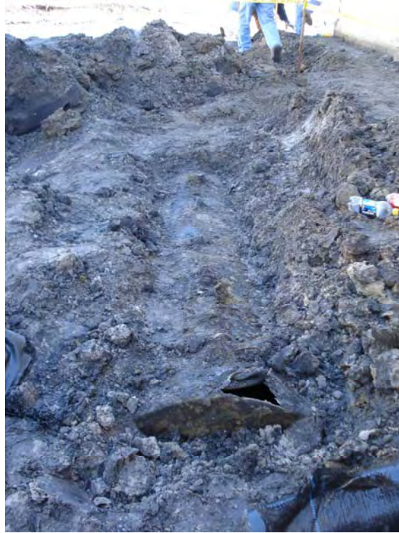
UST TT-3026 – Tarawa Terrace – Tank Exposed Pic #1 24Oct08
