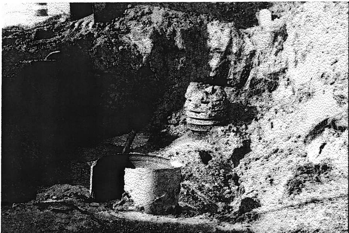
Photo 6 The fiberglass UST exposed. Note groundwater in excavation pit
