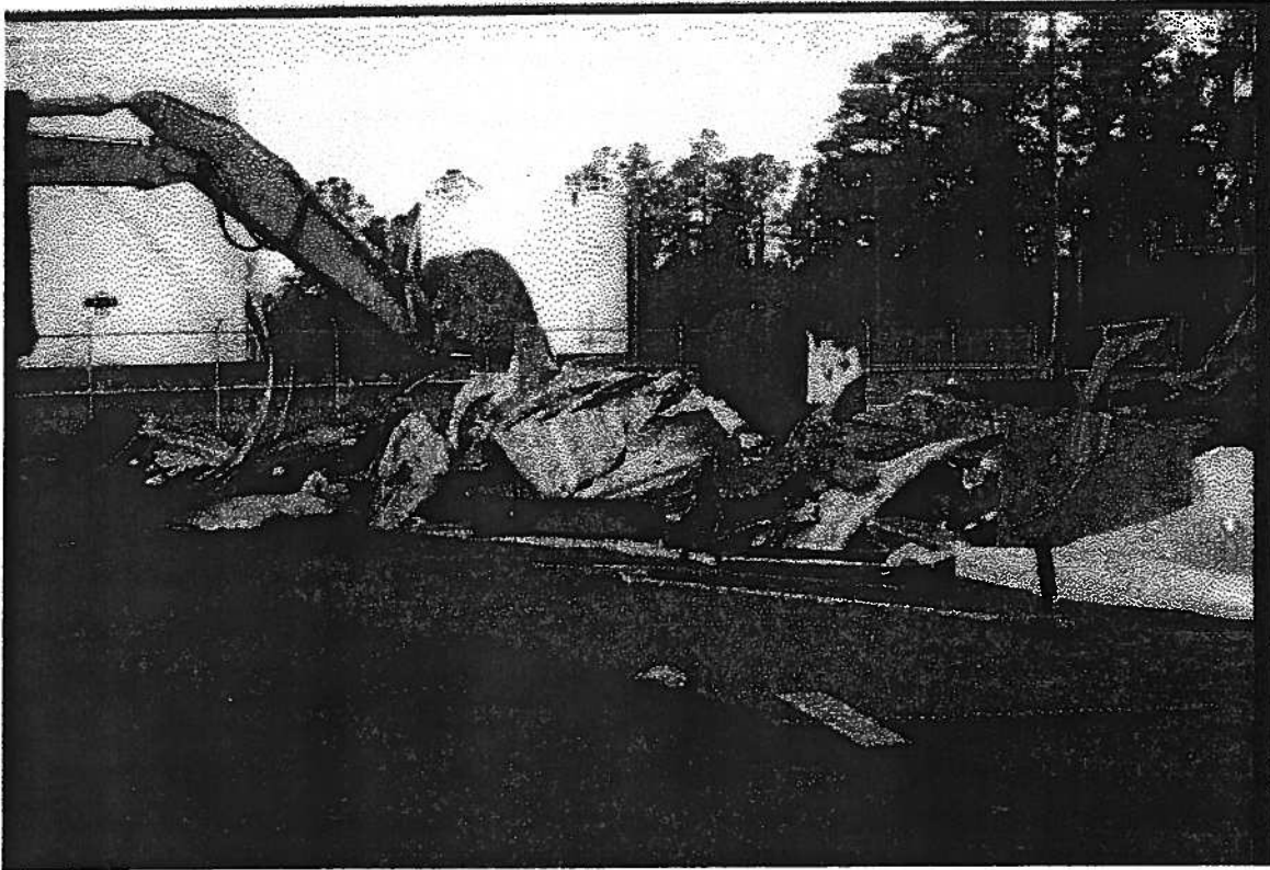
Photo 11 The UST is cut into pieces and ready to be transported to landfill
