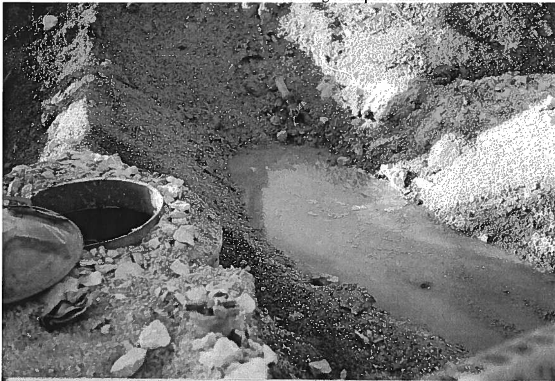
Photo #2 Groundwater in the excavation pit.
