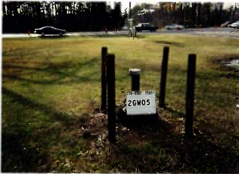
Figure 3-5 Shallow monitoring well 02-GW05 was also installed during the 1984 Confirmation Study. The well had begun to exhibit signs of neglect and deterioration.
