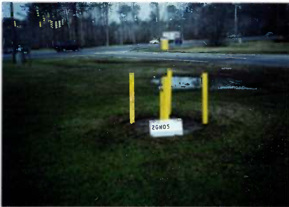
Figure 3-6 Peeling paint and rust were removed from the bollars and protective casing of shallow monitoring well 02-GW05. Two coats of weather resistant paint were then applied and a new padlock was installed.
