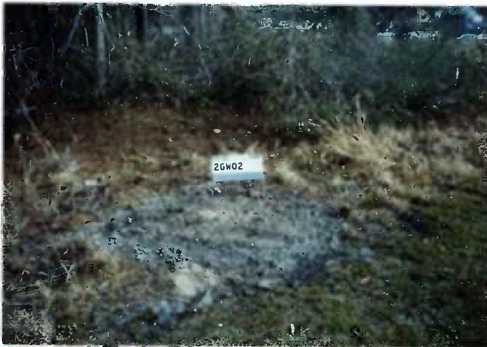
Figure 3-4 The pad, bollars, and protective casing of monitoring well 02-GW02 were removed. Topsoil and grass seed were used to restore the site.
