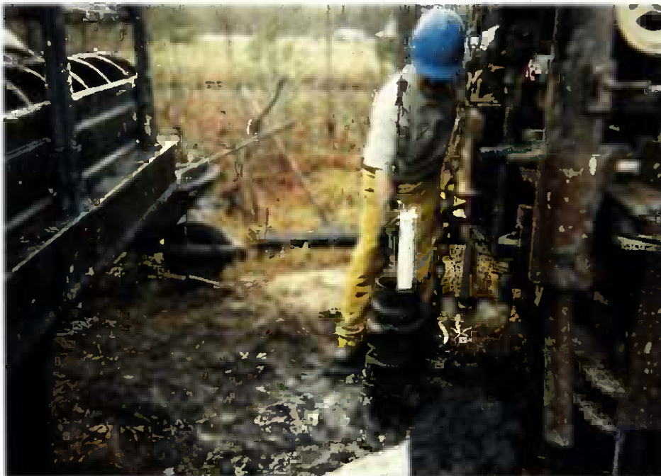
Figure 3-2 Two-inch polyvinyl chloride (PVC) well materials were used during installation of 02-GW03IW. Well construction materials were added to the annular space between the augers and PVC well.
