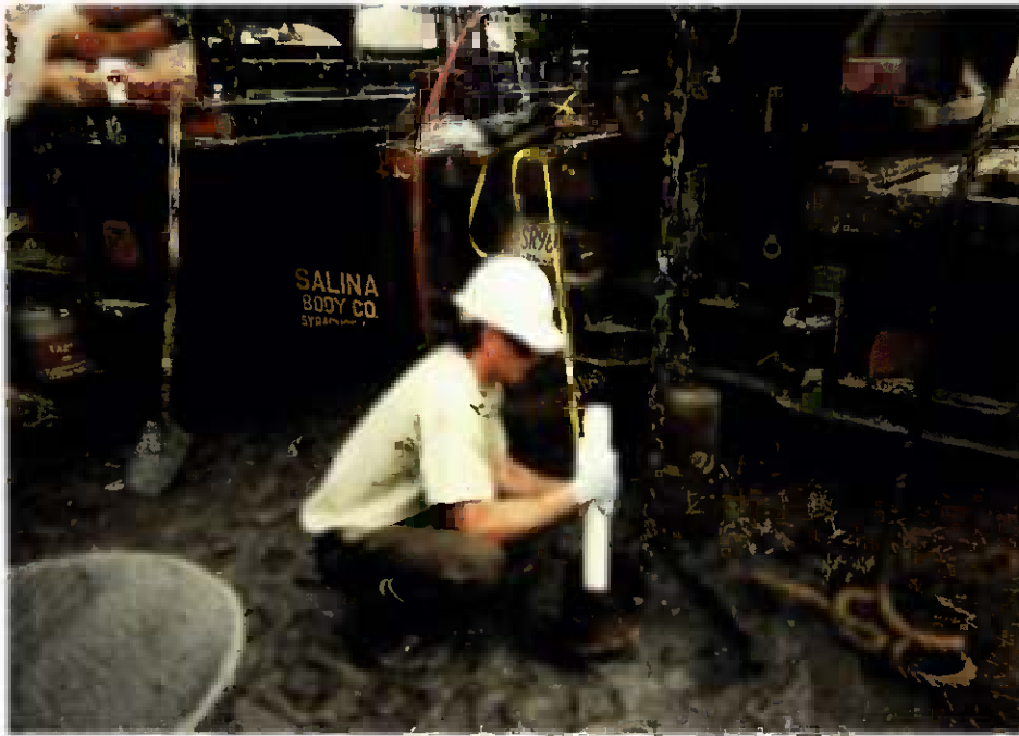
Figure 3-1 During well installation, 6-1/4-inch hollow stem augers were used as depicted here.
